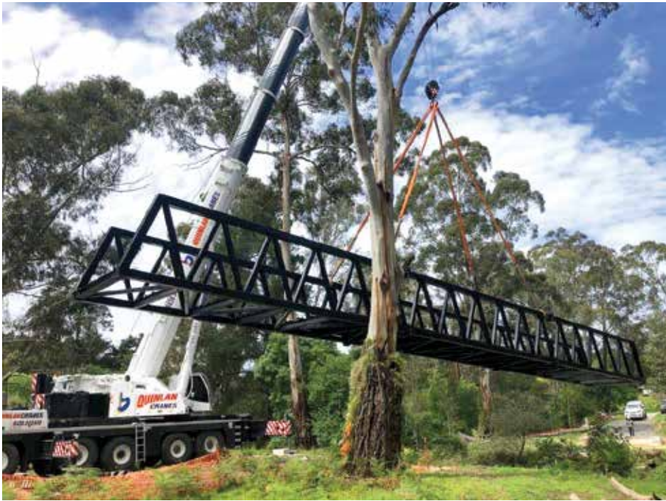
One of the five bridges is installed along the Diamond Creek Trail extension between Wattle Glen and Hurstbridge.
