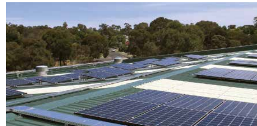
Community Bank Stadium's new solar photovoltaic panels
