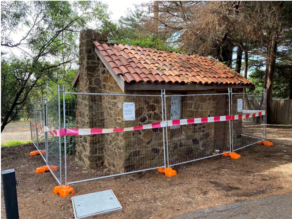
Stone caretaker's cottage hoarded off due to state of disrepair
