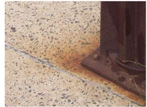
The effect of rusted metal on concrete - feature treatment for wall concept
