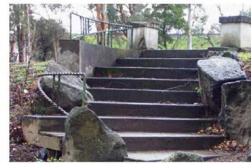
Existing metal work - Rusted Metal Reinforcing
