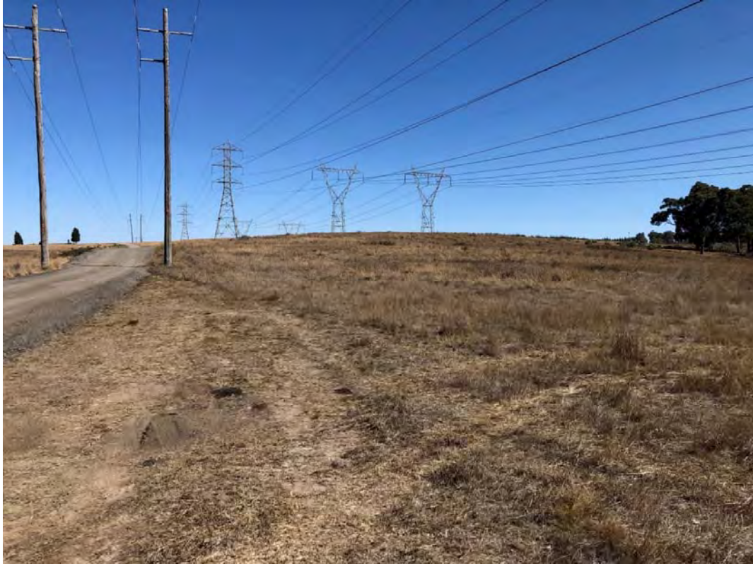
Photo 4: Hi-voltage transmission lines and towers which bisect the property at [REDACTED].
