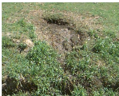
Figure 2: Blackwater leakage and pooling at Kent Hughes Road, Eltham
